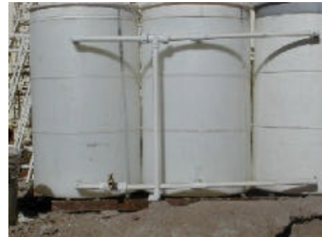
Figure 18 Hose Bib Attached to Cistern Piping
