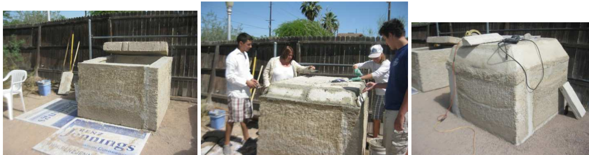
Figure 4.8. BARA student interns construct and discuss fibrous concrete test structures in Tucson, Arizona with CETis 128 teacher
