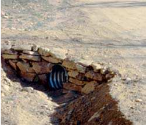
To be effective, culverts must be installed properly and at proper locations.
